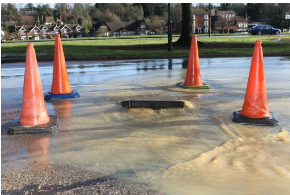
Photograph 8: A surcharged manhole (the sewer system has reached its capacity and water now escapes via manholes)
