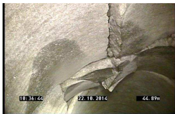
Image taken from a CCTV survey of a cracked and failing asset
