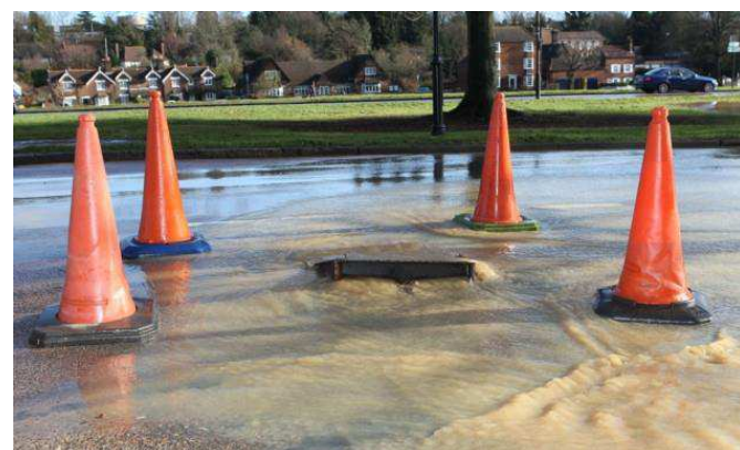
Surcharged manhole (the sewer system has reached its capacity and water escapes), Harpenden
