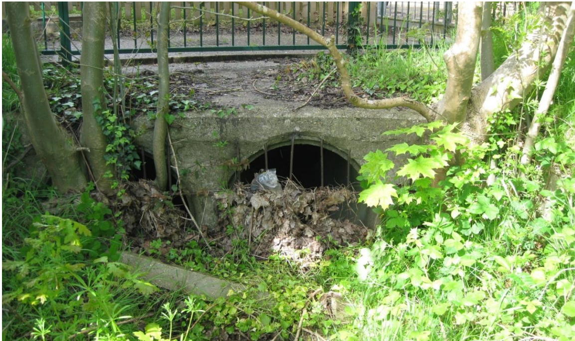
Photograph 5: Unmaintained culverts blocked by trees, plants & debris
