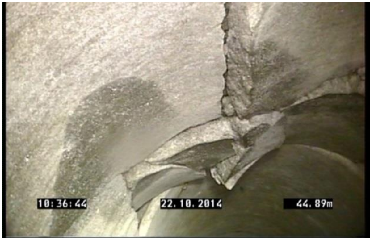
Photograph 17: Taken from CCTV survey of a cracked & failing asset
