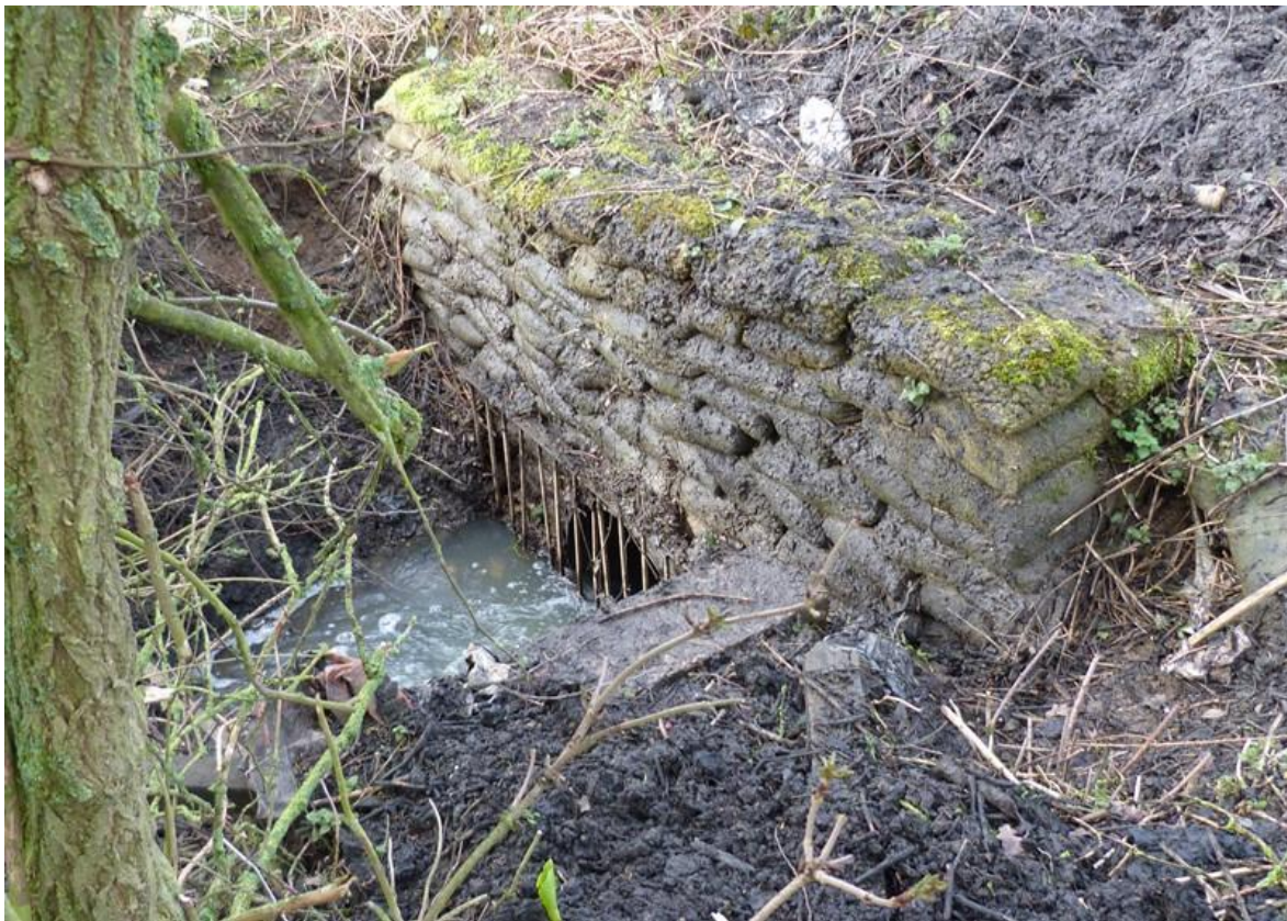
Photograph 15: Neglected and unsuitable structure in an Ordinary watercourse
