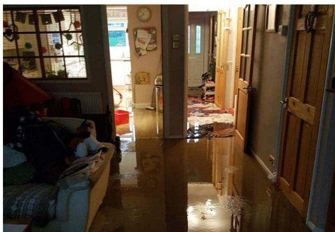
Internal property flooding
