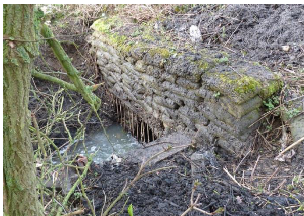
Neglected and unsuitable structure in an Ordinary Watercourse
